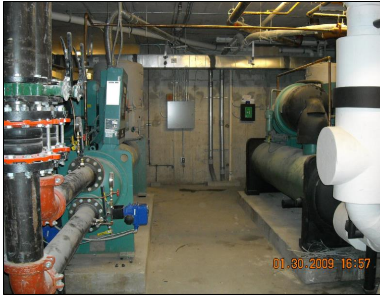
Untreated Screw Chiller
