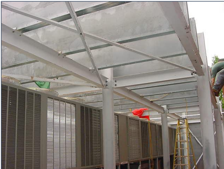
Roof Baffle Support Steel Spanning the Chiller
